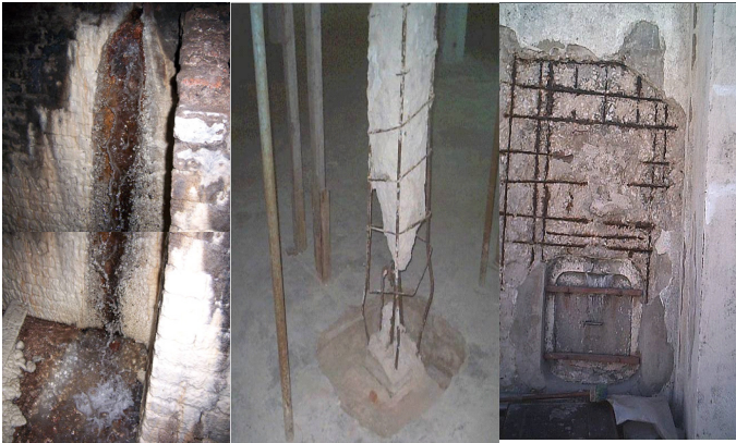
Figure 1. Basement flooding and damage of the reinforced concrete structures.
