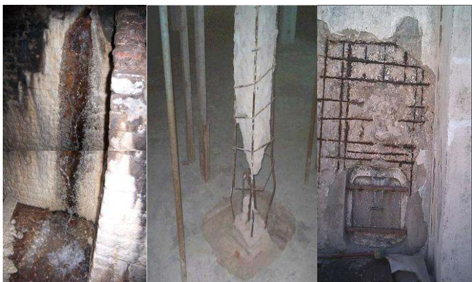
Figure 2. Basement flooding and damage of the reinforced concrete structures.
