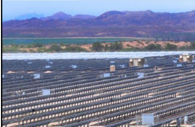
Yuma County, Arizona USA Agua Caliente Solar Project 247MWp (397MWp)
